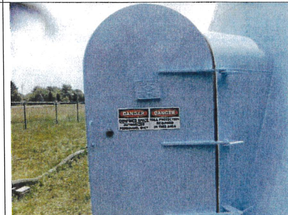
OSHA signs on the tank entrance door.
