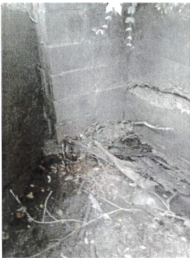
Drain Plugged up
