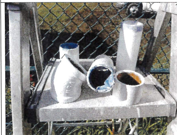
Painted pipe fitting for condensation drain.
